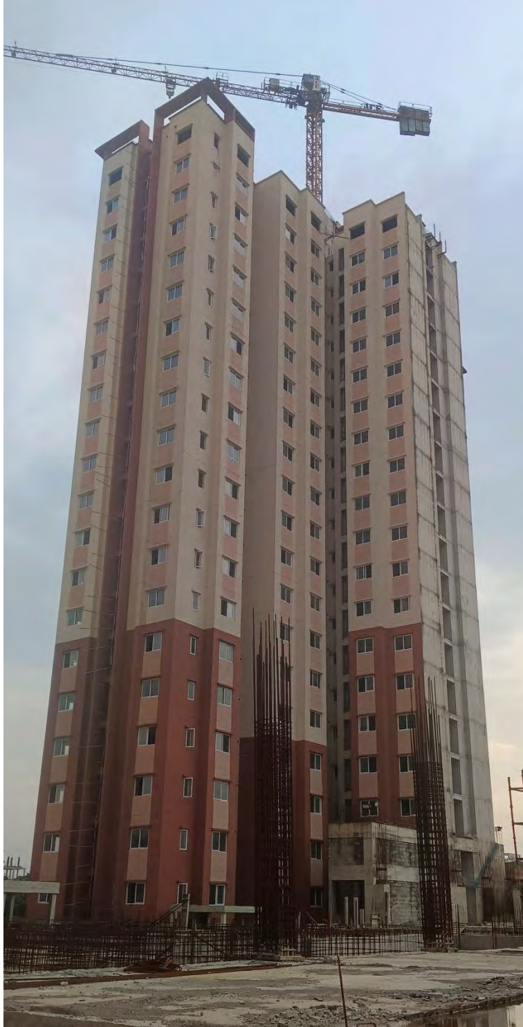
Terrace floor slab completed .Above terrace work and finishing work under progress
