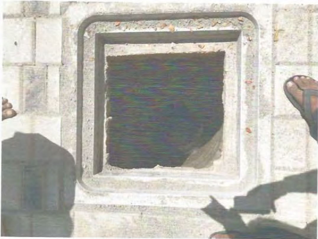
Rain water harvesting open & closed photos
